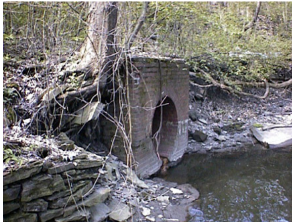
Sewer pipe dumping into the Willamette River
